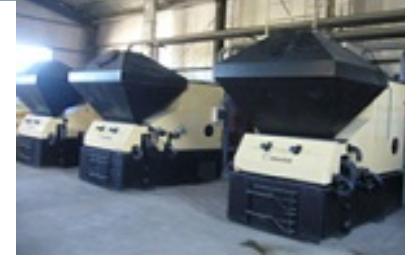
High-efficiency Heat only Boilers, Suuri-Keikaku, Mongolia
